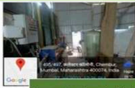
Sewage Treatment Plant
