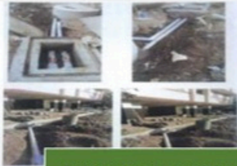
Rain water Harvesting
